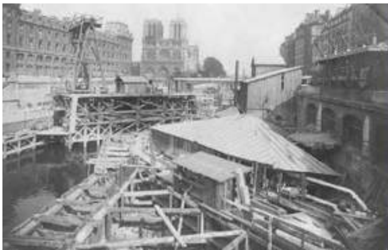
Installation de congélation en surface - Surface freezing installation
